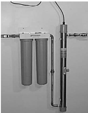
Completed installation with pre-filter set and UV. Inlet/outlet valves are recommended.
