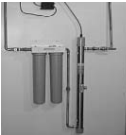
Completed Installation with Pre-Filter set and UV
